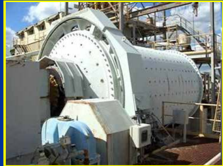
Typical Installation showing Covered Trunnion and associated Electric Motor
